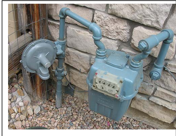
Figure 4: Natural gas shut-off valve located adjacent to the meter.
