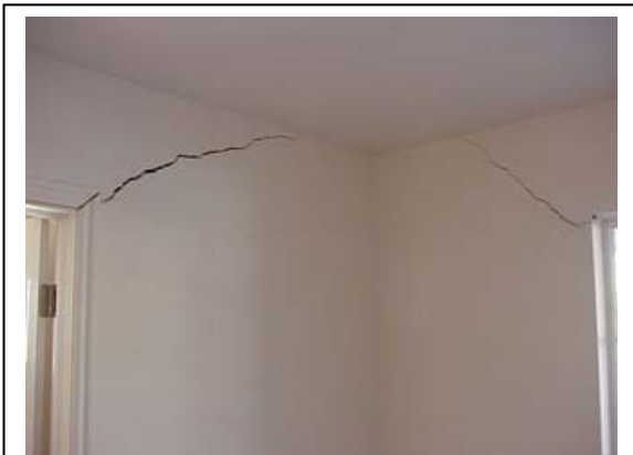
Figure 6: An example of large gaps in sheetrock
