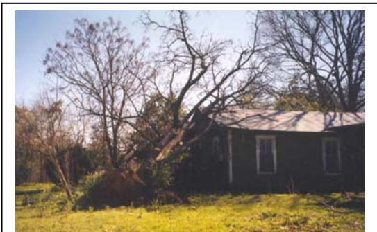
Figure 5: The weight of this tree could cause this part of the home to fall
