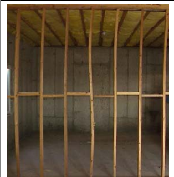
Figure 7: Notice the middle stud is deformed in an "S" shape.
