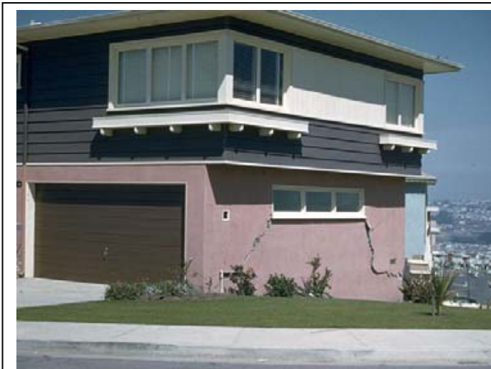
Figure 1: Cracks in a masonry are a sign of danger.
