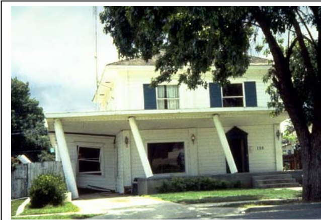
Figure 3: Leaning porch after an earthquake
