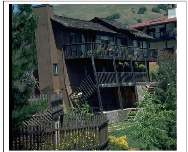
Figure 2: Notice the entire wall near the chimney is out of plumb.
