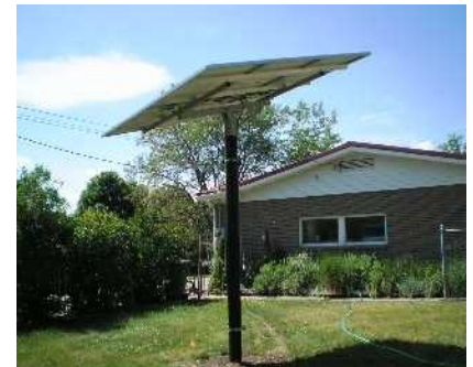
Charles Ashurst's Photovoltaic system in Logan, Utah
